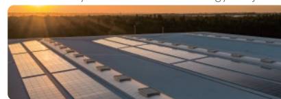
工业园区光储充微电网 Photovoltaic storage charging microgrids in industrial parks
